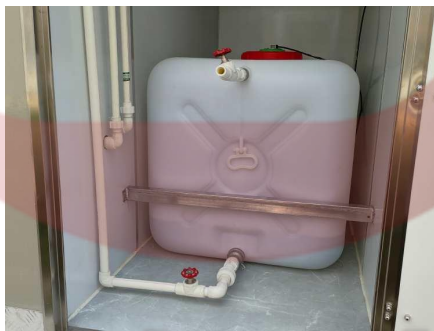
- Clean Water Tank -
